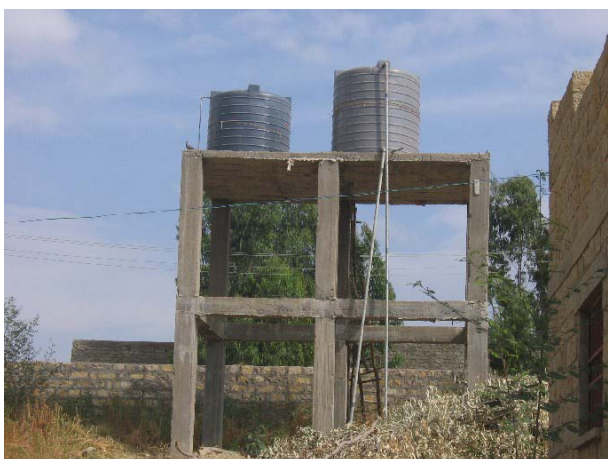
The New Water Tanks
